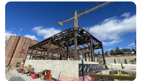
At Wellspan Health Surgical and Critical Care Tower, the concrete mix designs utilized type 1L cement, and steel column sizes were reduced through the use of 65ksi steel.
